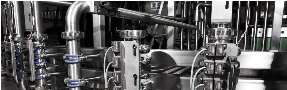
Piggable Liquid Transfer and Distribution System
