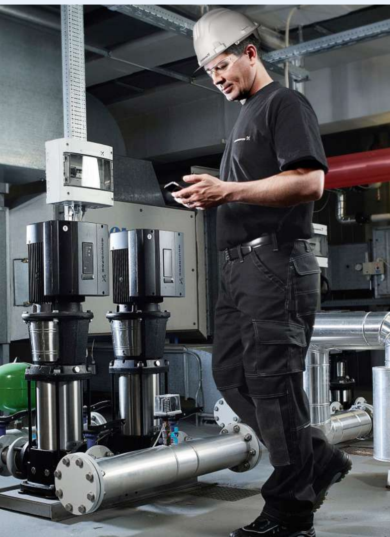
Figure 2: You can only improve something if you’re able to measure it. After all, you can only monitor operating states, optimise processes and thus exploit potential energy savings if you have subjected your system to rigorous measurement.
