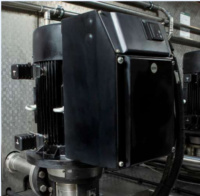
Figure 8: Regardless of the sector the operator is active in, Grundfos Machine Health can offer real benefits in any installation. The solution provides user-friendly, actionable insights that help users anticipate problems before they lead to outages.
