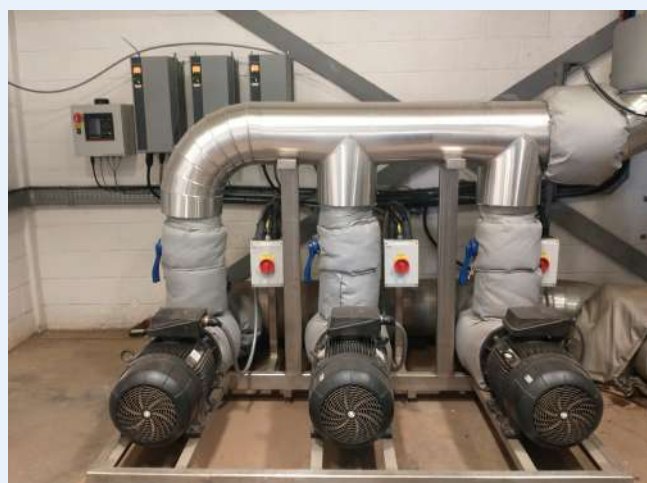
Figure 7: The Grundfos team advised Arla Foods on the selection of smart pumps and controls, and delivered a turnkey end-to-end system for cooling and ice water. This included the installation, pipework and commissioning, and validation of the savings.
